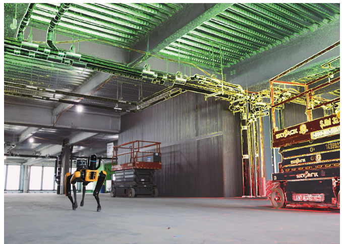
Spot streamlines Turner's ability to perform laser scans and document as-built conditions.
